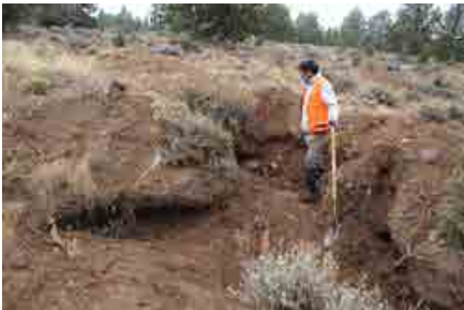
Dig site requiring remediation.
