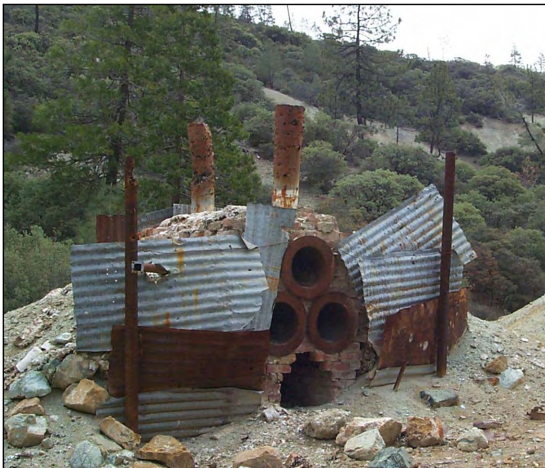
Figure 3.13-6: Xanadu Millsite prior to Abandoned Mine Lands clean-up (T. Moore, USDI BLM).
